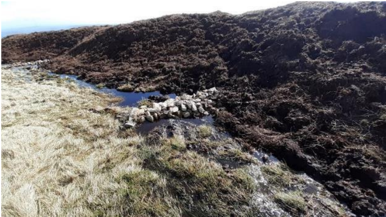
Photo 2 Stone baffles used to slow down the flow of water and protect the toe of the reprofiled slope. This gully is 2m high.
