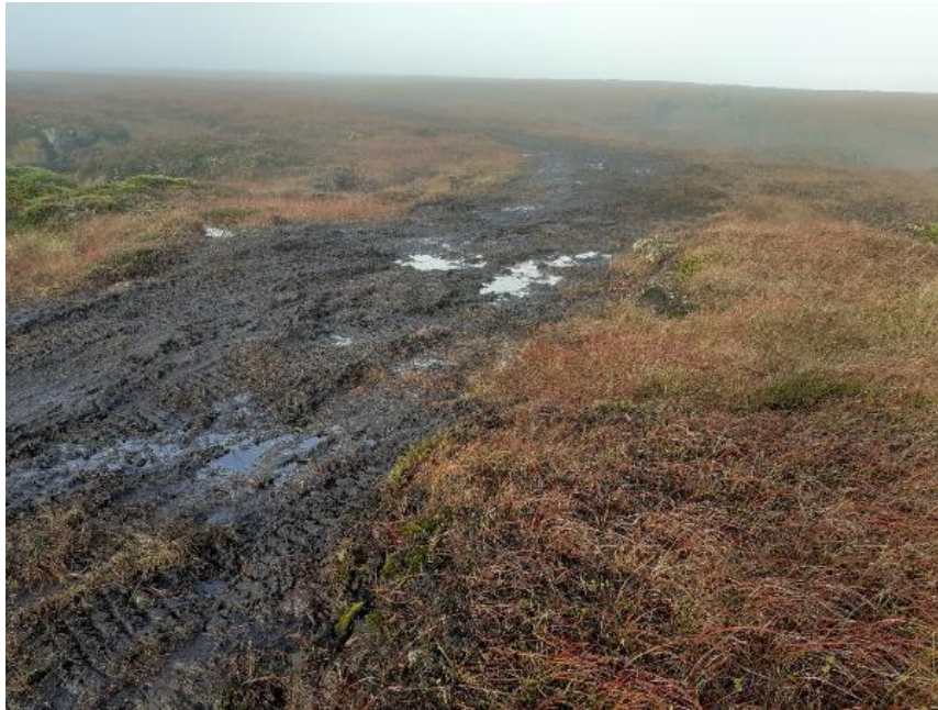
Figure 3 Photo showing increased surface disturbance and if not repaired could show visible signs of tracking after 12 months.
