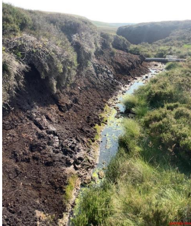
Photo 4 Photograph showing typical location for stone dam proposed for protection of re-profiled gully side at Snailsden (gully side shown prior to re-profiling).
