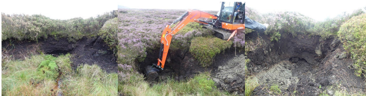
Fig. 8. Photographs showing preparation for blocking within a collapsed pipe “gully” section
