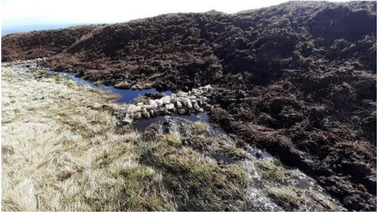
Photo 2 Stone baffles used to slow down the flow of water and protect the toe of the reprofiled slope. This gully is 2m high.
