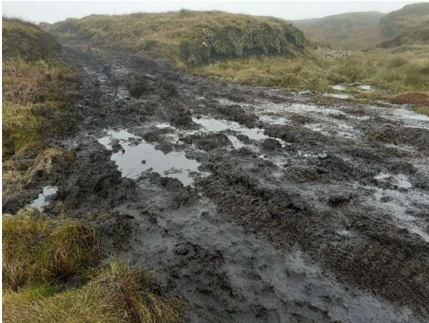
Figure 4 Photo showing access route in bad condition and if not repaired would still show visible signs of tracking within 12 months.
