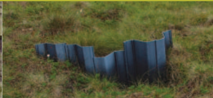
Blocking drains with plastic dams to rewet heather dominated bog. This may be all that is required but monitoring is required to confirm that a rise in the water table is then controlling heather growth and allowing an expansion of sphagnum
