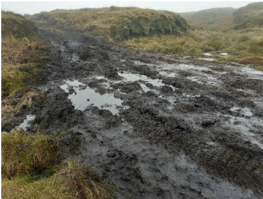
Figure 4 Photo showing access route in bad condition and if not repaired would still show visible signs of tracking within 12 months.
