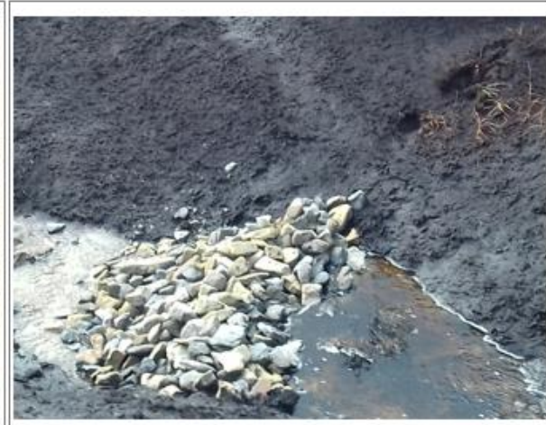
Gully blocks - Channels are blocked to retain water in the habitat and help restore the sites hydrology
