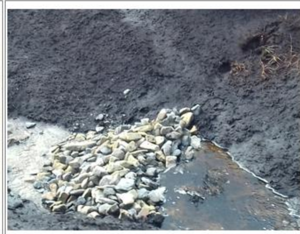
Gully blocks - Channels are blocked to retain water in the habitat and help restore the sites hydrology
